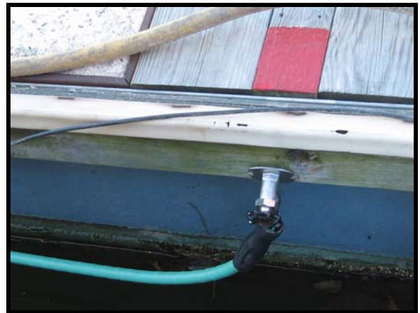
A hose temporarily connected to a "Winter Water" spigot
