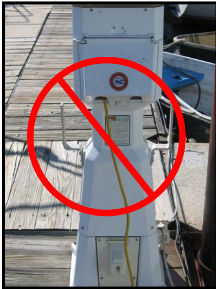
120V extension cord plugged into 120V outlet on power pedestal
