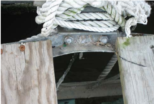
'K' Dock angle iron damage
